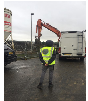
One of our Year 11's working on a local construction site in Burnley!
